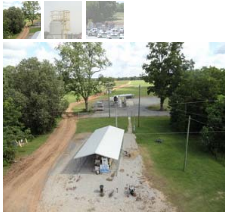
This is a view of the St. Landry Parish Solid Waste project's gas collection system to the BioCNG fueling station, which currently provides 150,000 DGE per year. Angela Cutrera, St. Landry Parish Solid Waste.
