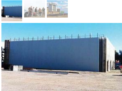
CR&R Environmental Services is implementing German-based Eisenmann's biogas technology for its project in Perris, California. The high-solids anaerobic digestion system employs a continuously fed, horizontal plug flow design. PHOTO: CR&R ENVIRONMENTAL SERVICES
