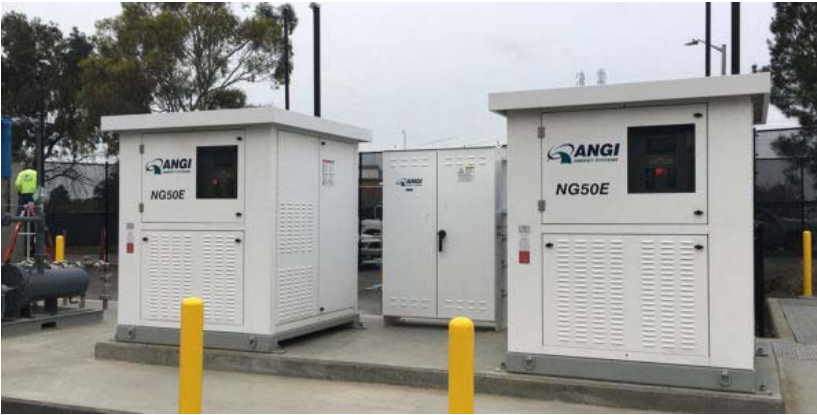
ANGI compressor units for the City of San Mateo, Calif.
