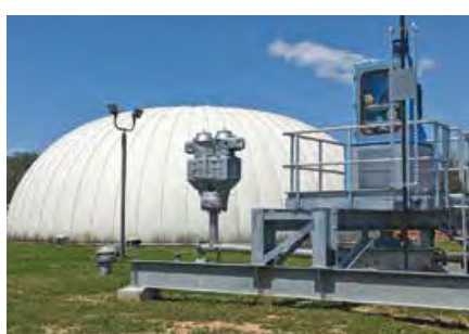
Digesters were upgraded and new mixers added when the Western Virginia Water Authority began converting its biogas to renewable natural gas.
