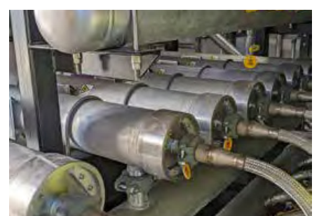
Membrane filters are part of the Unison Solutions system to convert biogas to renewable natural gas.
