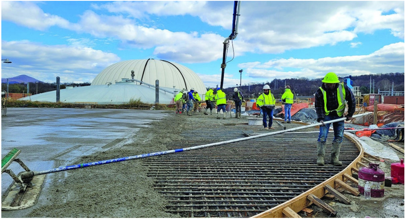
Workers spread concrete for a new digester at the Roanoke Regional Water Pollution Control Plant.
