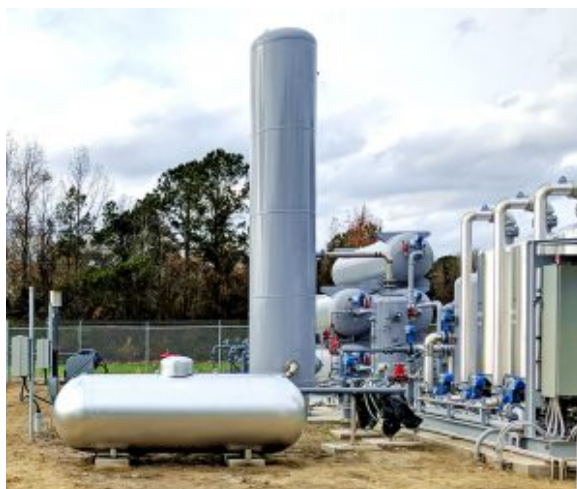
The biogas upgrading system at Optima KV consists of pressure-swing absorption to remove CO 2 , H 2 S and other constituents. Cleaned biomethane is pressurized to be sold to Duke Energy via its subsidiary, Piedmont Natural Gas. Photo courtesy of Cavanaugh
